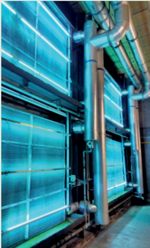
UVC Sanitisation of T3 Air Handling Unit cooling coils – this inactivates virus and irradiates the cooling coils to reduce mold and bacteria growth on its wet surface
