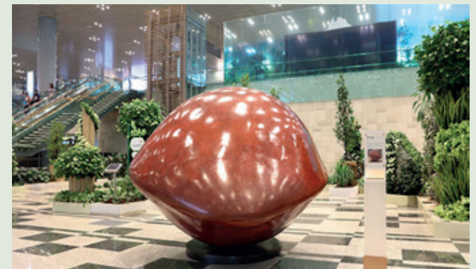
Terminal 3 Arrival Immigration areas are pleasantly cooled by AHUs with EC FanGrids
